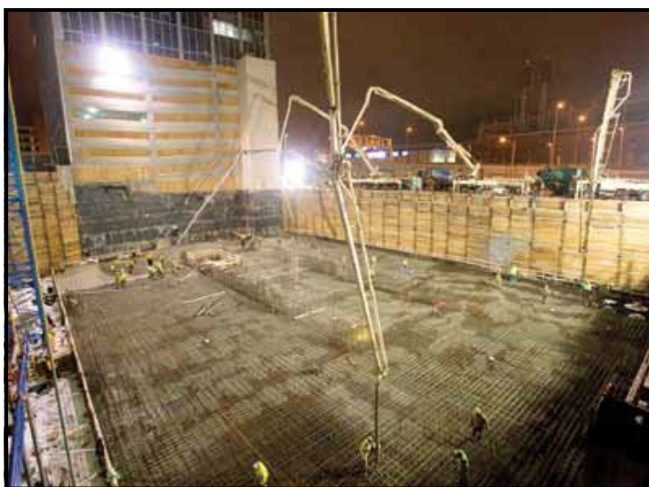
Fig. 4: The mat foundation placement on a Sunday morning. Ambient temperatures were between 25 and 30°F (-4 and -1°C)
